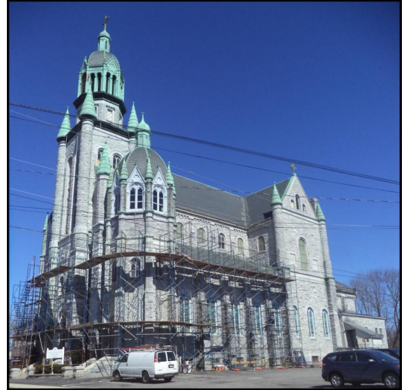
Repairs are under way at the St. Mary and Archangel Michael Church in Nashua.
